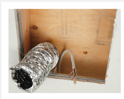
Existing 3" duct and wiring
